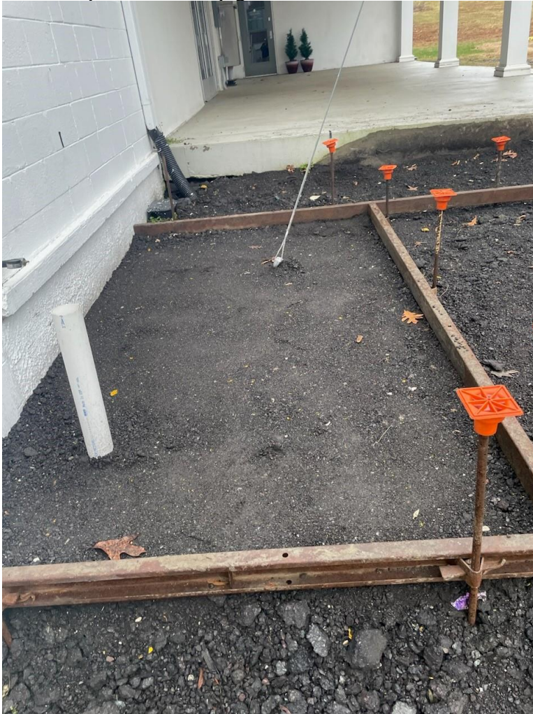
Concrete pad for back-up generator
