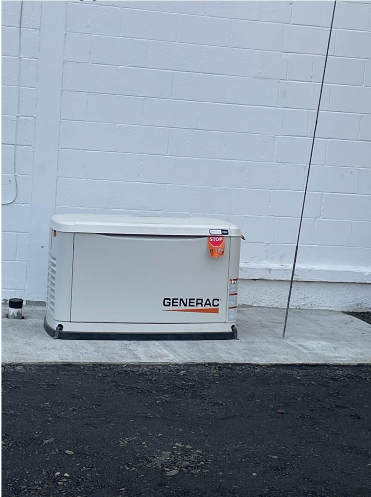
GBC back-up generator
